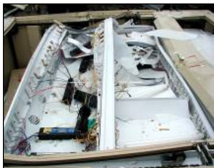
Prohibited: Ballasts on light fixtures in x-ray film reader
