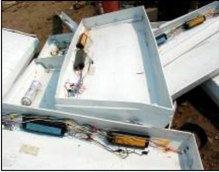
Prohibited: Ballasts on fluorescent light fixtures
