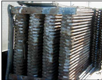
Prohibited: Heat exchanger with deposit / scale
