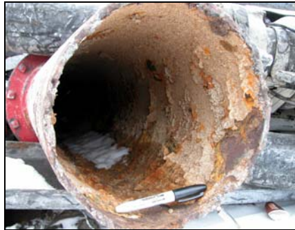
Prohibited: Pipe with radioactive deposit / scale
